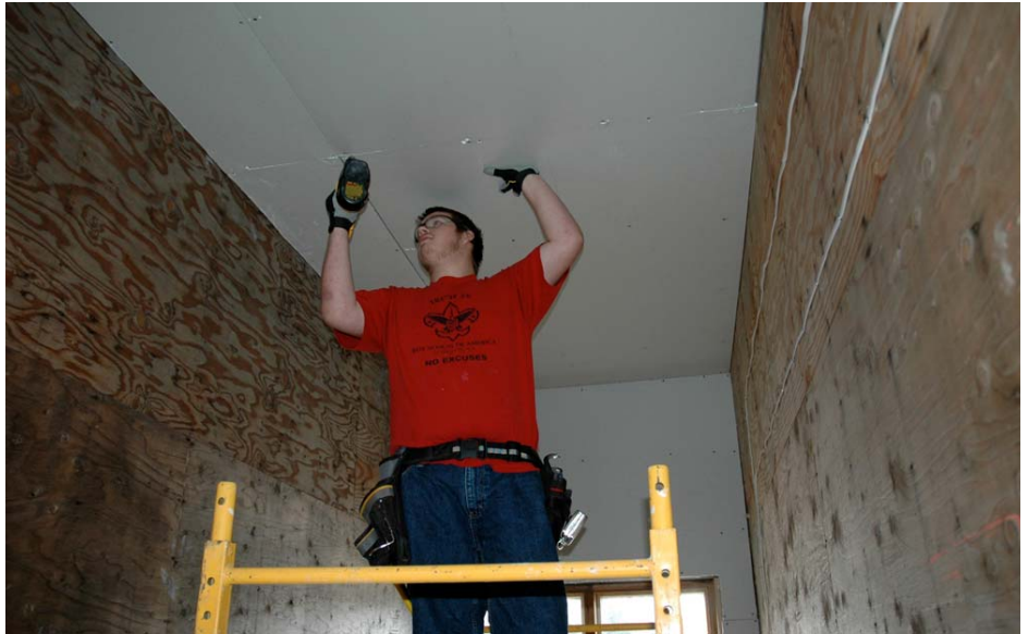
ABOVE: Andy Sulkowski puts up sheetrock in the Habitat for Humanity house.
